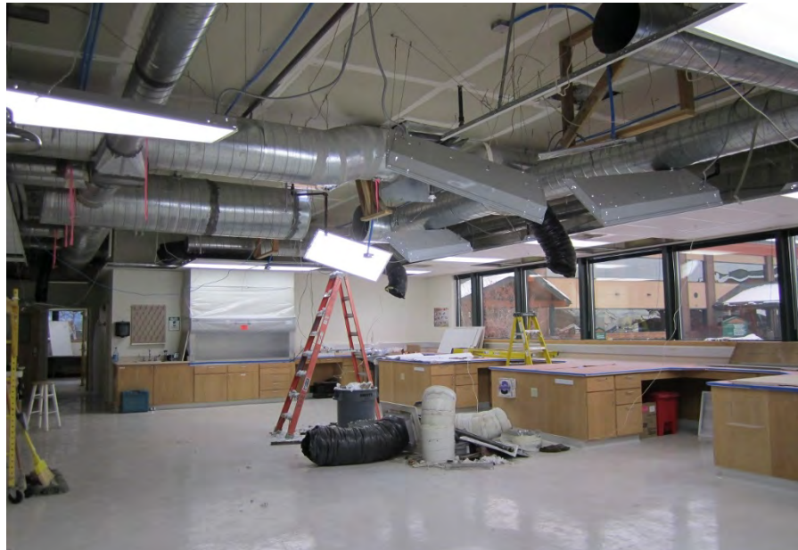
The DNA/serology section during HVAC renovations
