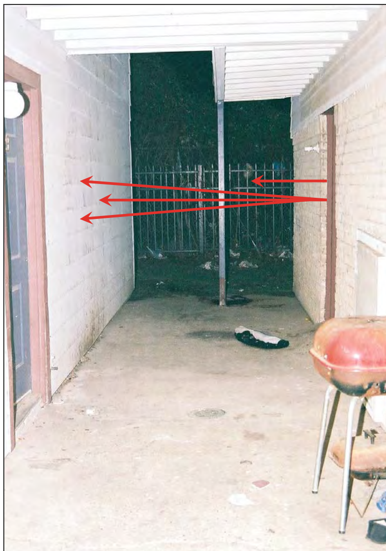
Figure 1-Four shots (red arrows) were delivered from the interior of the apartment on the right. One fired bullet struck an individual and was stopped; the other three impacted the wall across the corridor.
